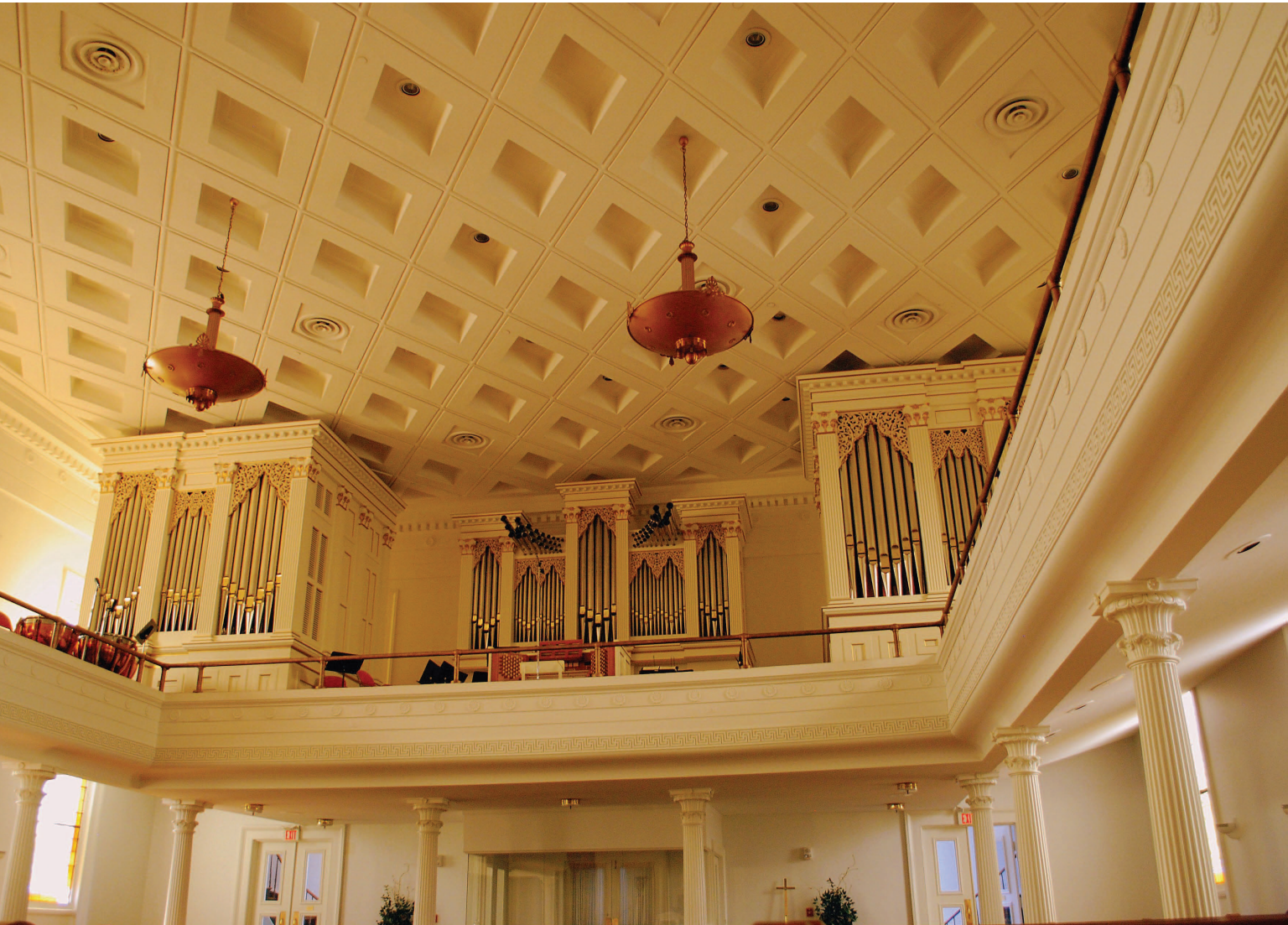
The main auditorium features a deeply coffered diamond-pattern ceiling and a pipe organ occupying the full rear balcony.
